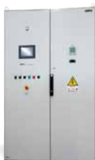
Automation and control board QPR
